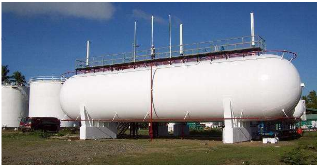
ABOVEGROUND PRESSURE VESSEL
