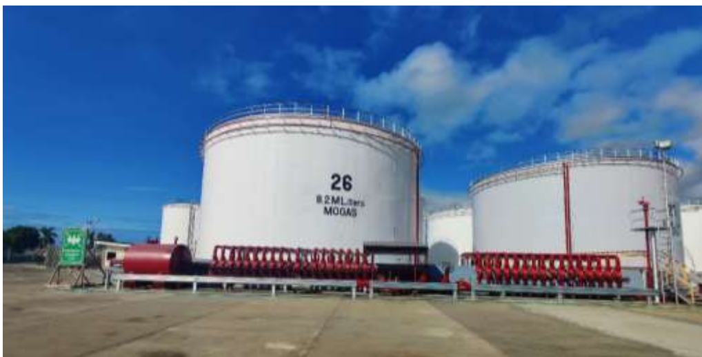
VERTICAL STORAGE TANK
